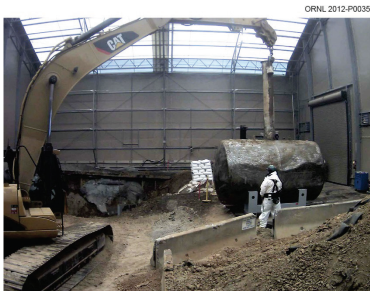
Fig. 5.42. Removal of Tank W-1A eliminated the main source of groundwater contamination at Oak Ridge National Laboratory.
